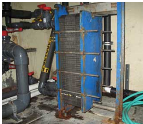
Figure 2. Ten titanium heat exchangers are located throughout the facility, allowing specific seawater temperatures to be maintained throughout the 18,000 square feet of wet-lab space.
