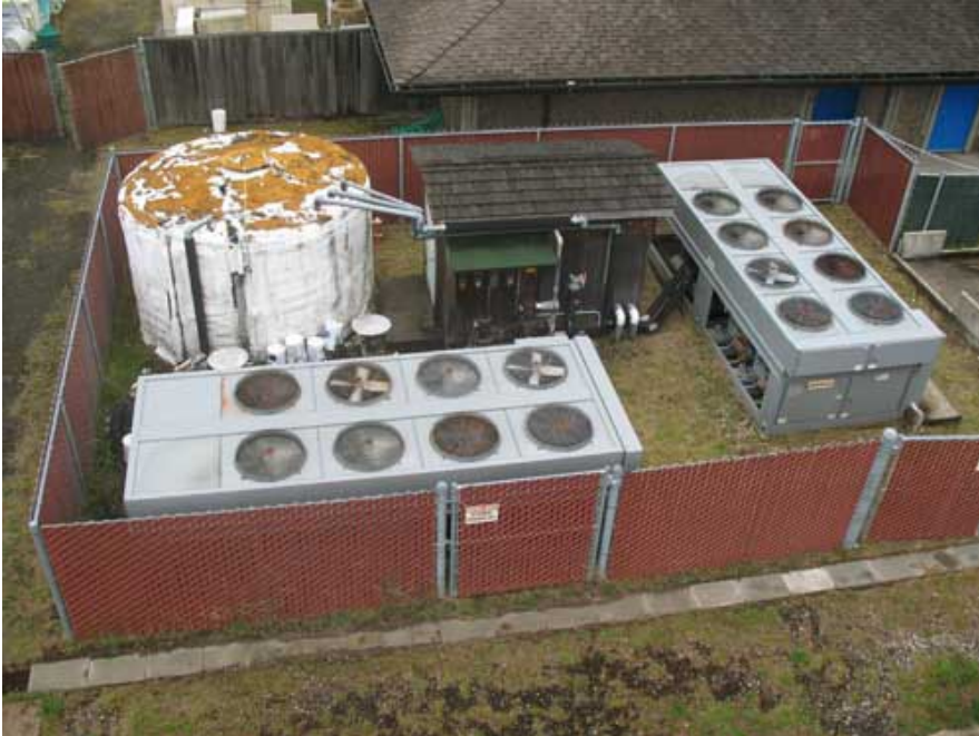
Figure 1. The seawater chilling plant consists of two 100-ton chilling units that continually cool and recirculate glycol through a 5,000-gallon reservoir. From the reservoir the glycol is pumped to exchangers throughout the facility in order to chill seawater.
